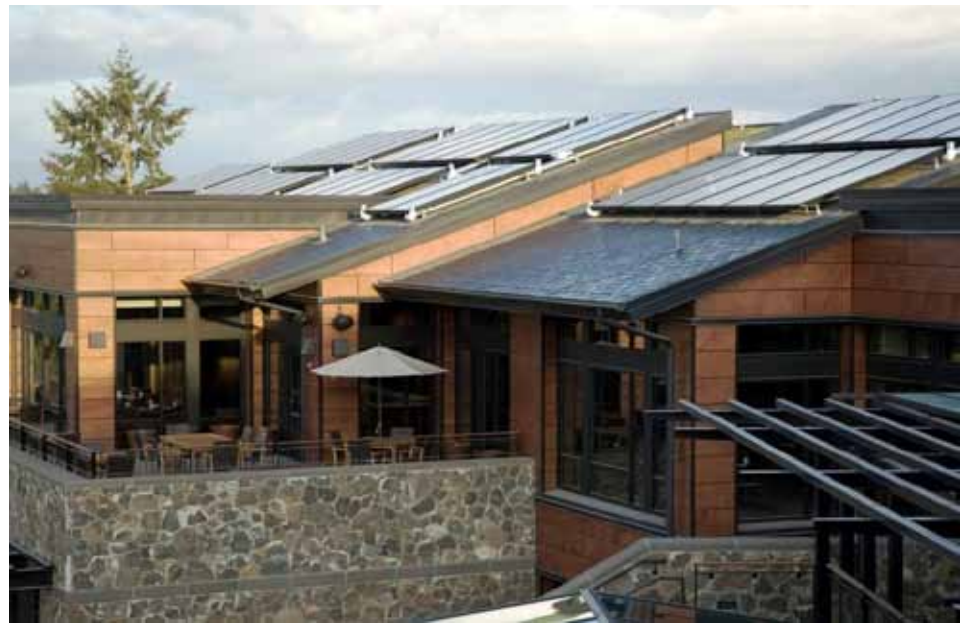
Solar thermal installation at the Allison Inn, Oregon
