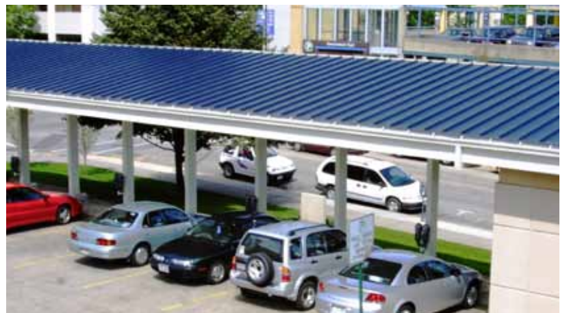
Photovoltaic awning at parking structure in Madison, Wisconsin
